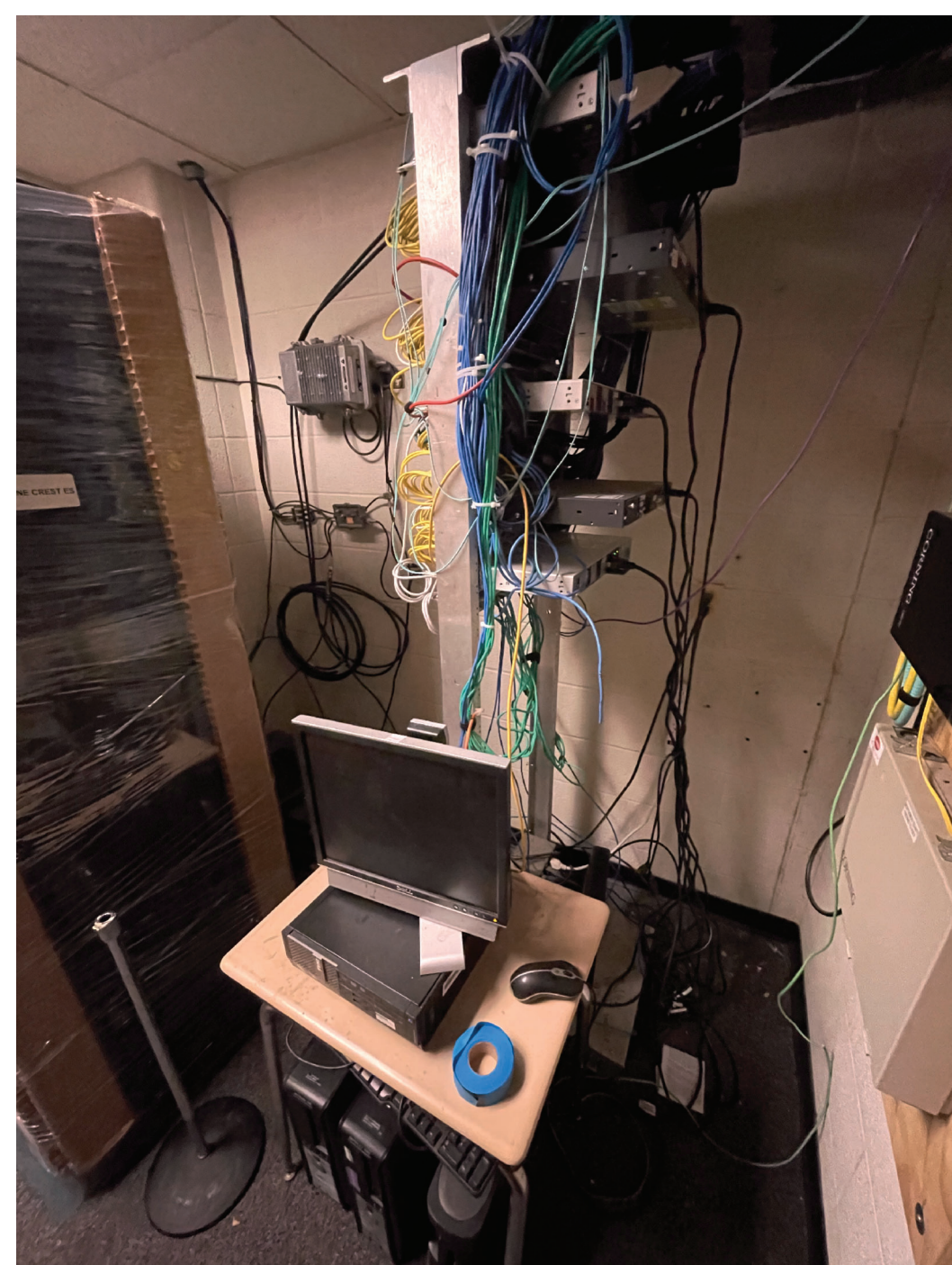
3 MAIN BUILDING IT ROOM
